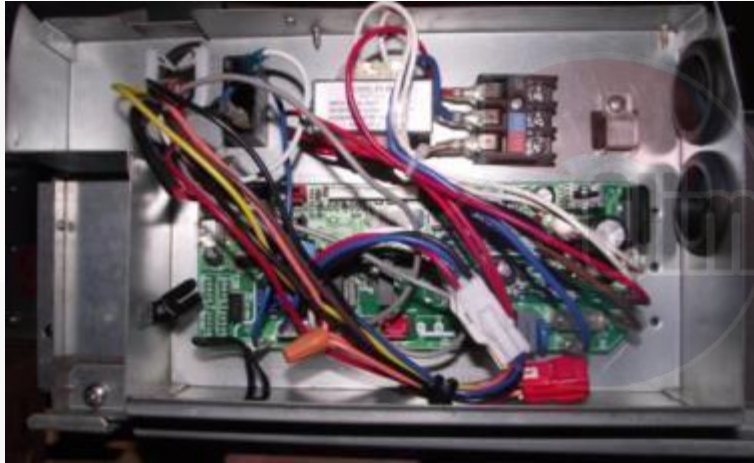
Indoor control board
