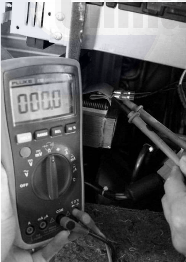
Fig. 36 – Reactor resistance test
